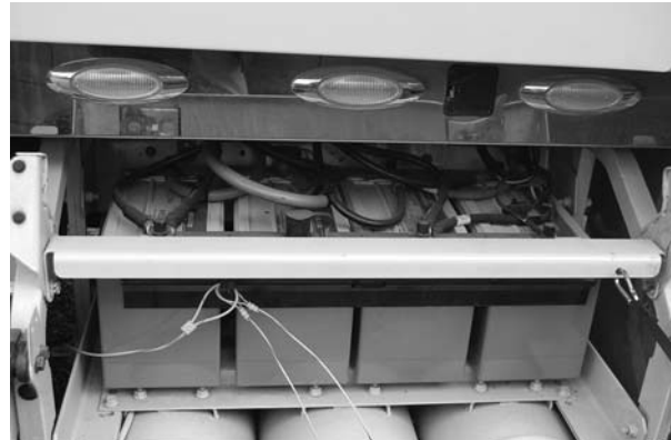
Figure 1 – AGM batteries replace standard lead-acid batteries
